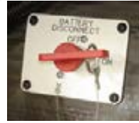
Battery Disconnect Switches
