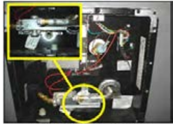
Fig 1: Water heater drain plug
